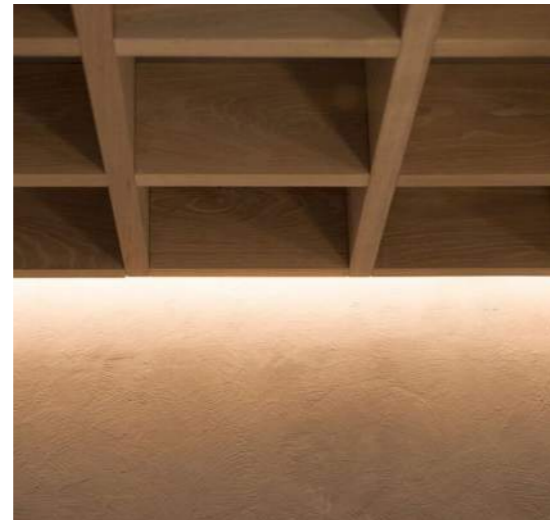
Acoustic Ceiling Grid
